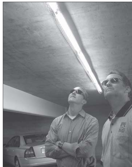
Public Services analyst Matt Huffaker, left, and Building Maintenance Supervisor Steve Schmidt inspect the new, energy-efficient lighting in the North Locust Street parking structure.
