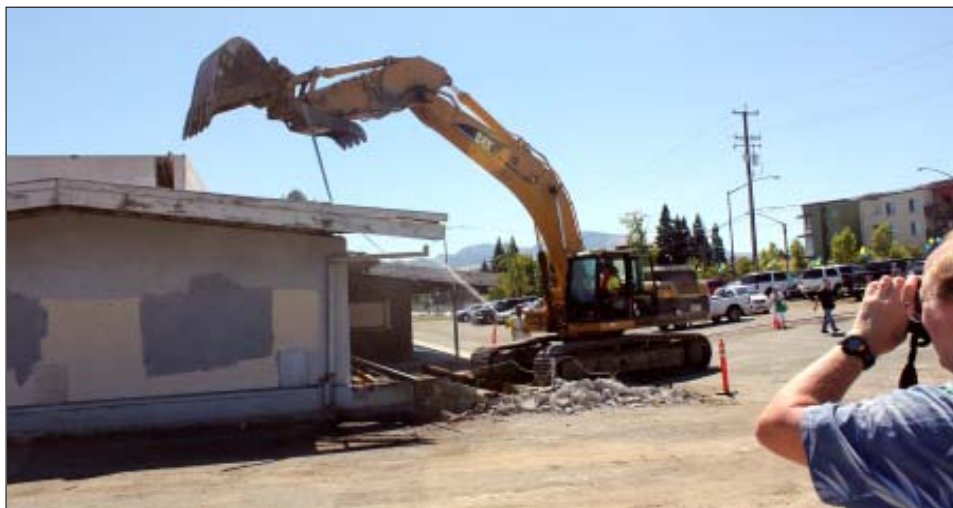
END OF AN ERA — A bulldozer takes a big bite out of the old co-op at Geary and North Main to make way for a new project known as the Geary Marketplace, which will feature a Sprouts Farmers Market grocery store, a Habit Burger restaurant, SuperCuts and The Coffee Bean & Tea Leaf cafe. The marketplace is expected to open in Spring 2012.
