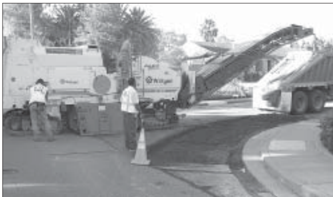
Street resurfacing projects throughout Walnut Creek, and particularly in the downtown, accounted for the lion's share of Capital Improvement Program (CIP) funding in 2005 and 2006. (For details about the City's street maintenance program, see page 16.)
